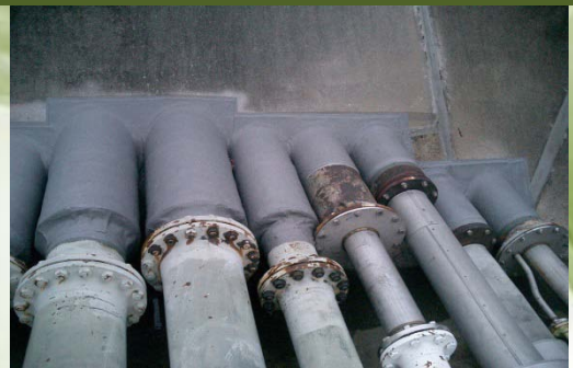
Elastische Einbindung von Rohrtrassen in WHG-Flächen Elastic integration of pipeways in areas subject to the German Water Resources Act (WHG)
